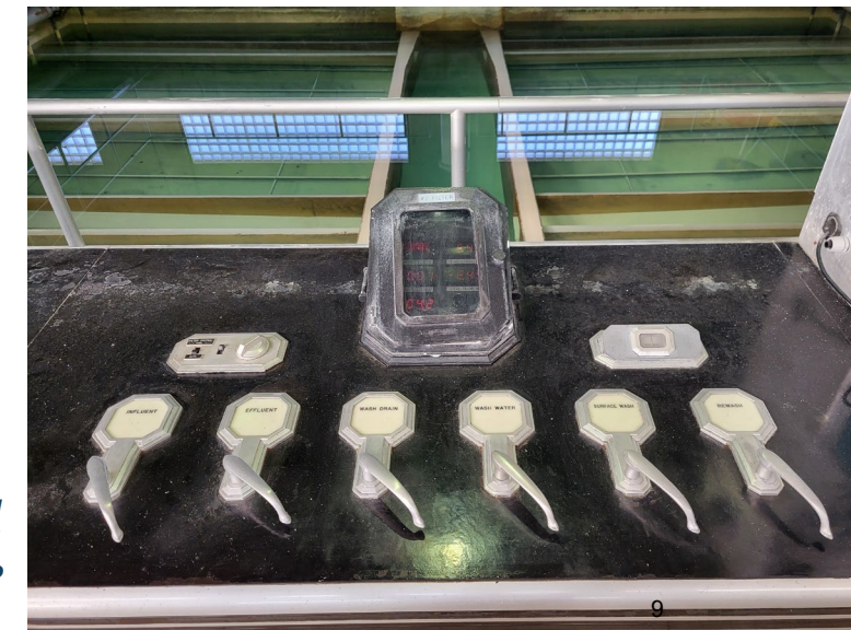
Filter Control Console
