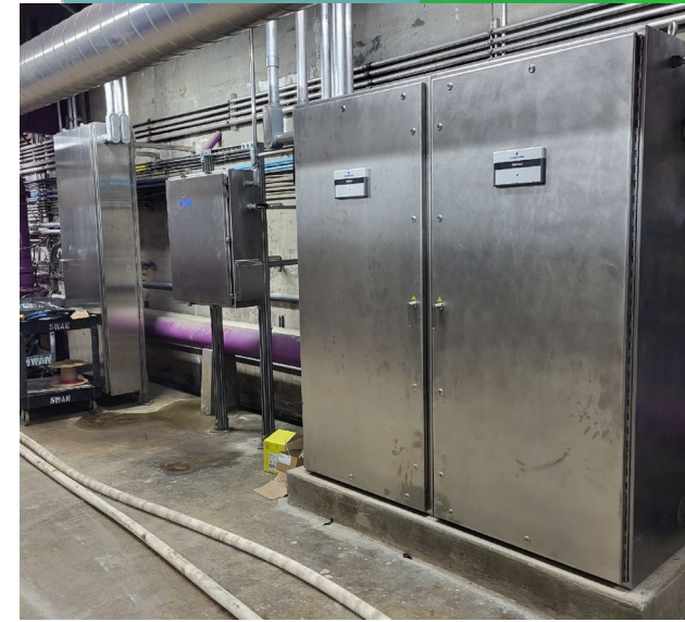
New Filter Control Panels to be integrated and connected to the filter operation system in Fall of 2024
