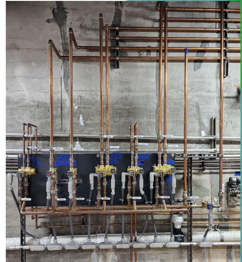
New solenoid valve configuration replaces cluttered, hard-to-access valves
